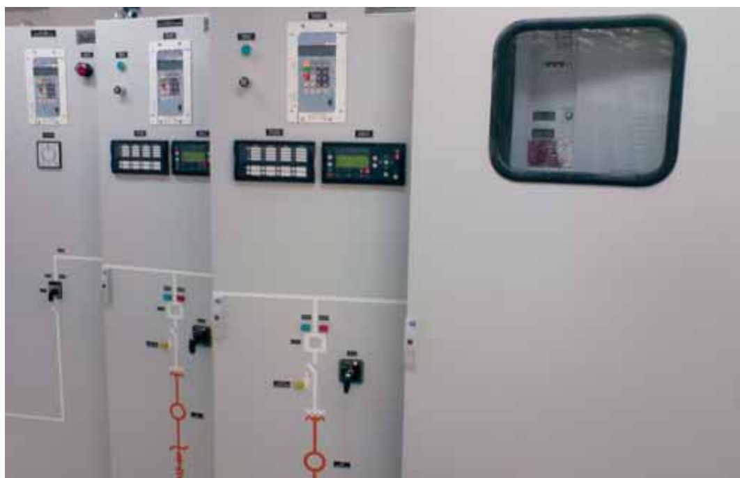
› smART P500 in cubicles.
